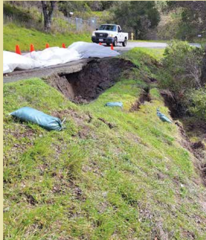
Sawyer Camp Trail remains closed as it has suffered a lot of damage from the storms. Earth is sliding out from underneath the trail in multiple
