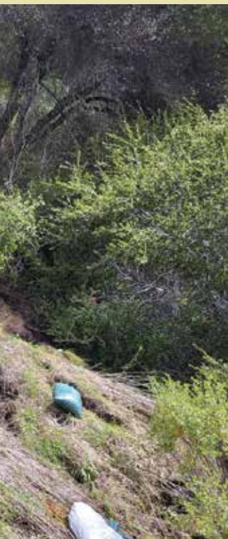
Damage from our back-to-back fire locations causing instability.
