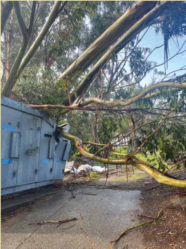
Power is down for everyone at Coyote Point thanks to this culprit.
