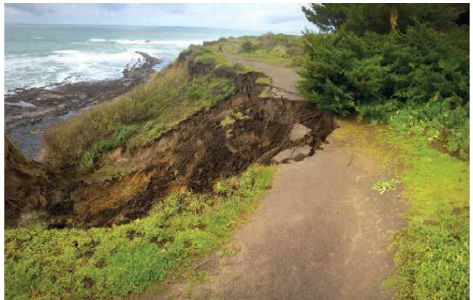
Erosion on trail at Pillar Point bluff.
