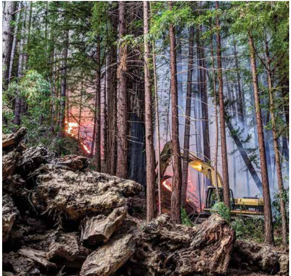
A San Mateo County Park Ranger operates a masticator to create a fuel break.
